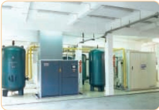
Nitrogen Generator for Lead Free Soldering
