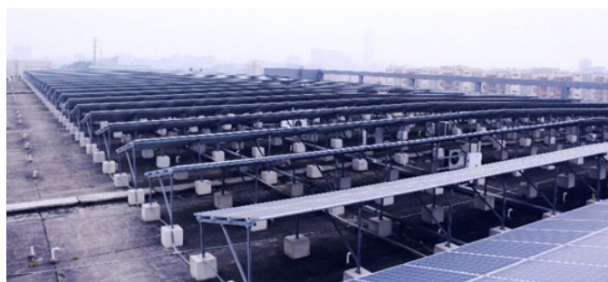
Solar photovoltaic power station
